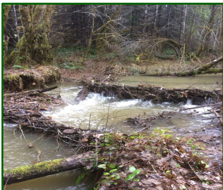
Some constructed BDA's utilized a double back to back design to reduce lift heights
