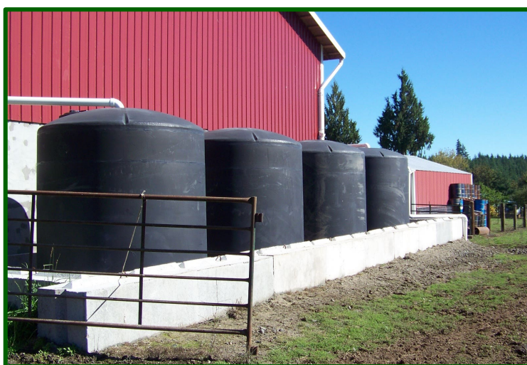
New roof run-off system with storage tanks that will provide water for livestock troughs
