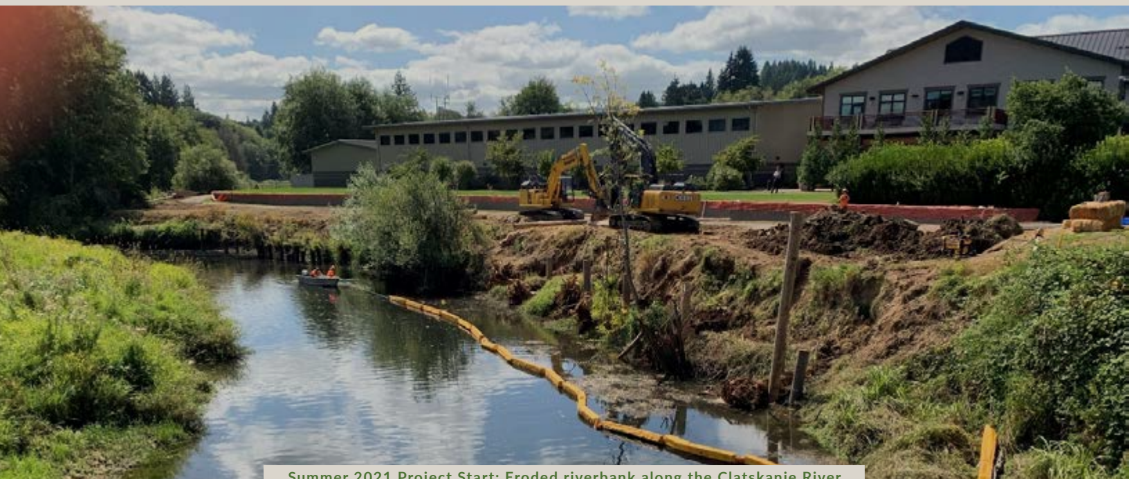
Summer 2021 Project Start: Eroded riverbank along the Clatskanie River that was slumping into the channel
