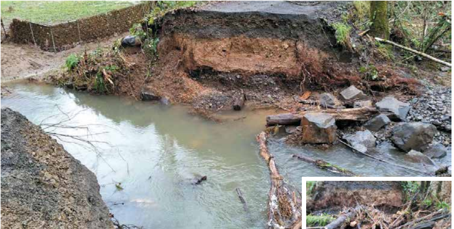
Hills Haven Road in ruins after the culvert blew out in December 2015.
