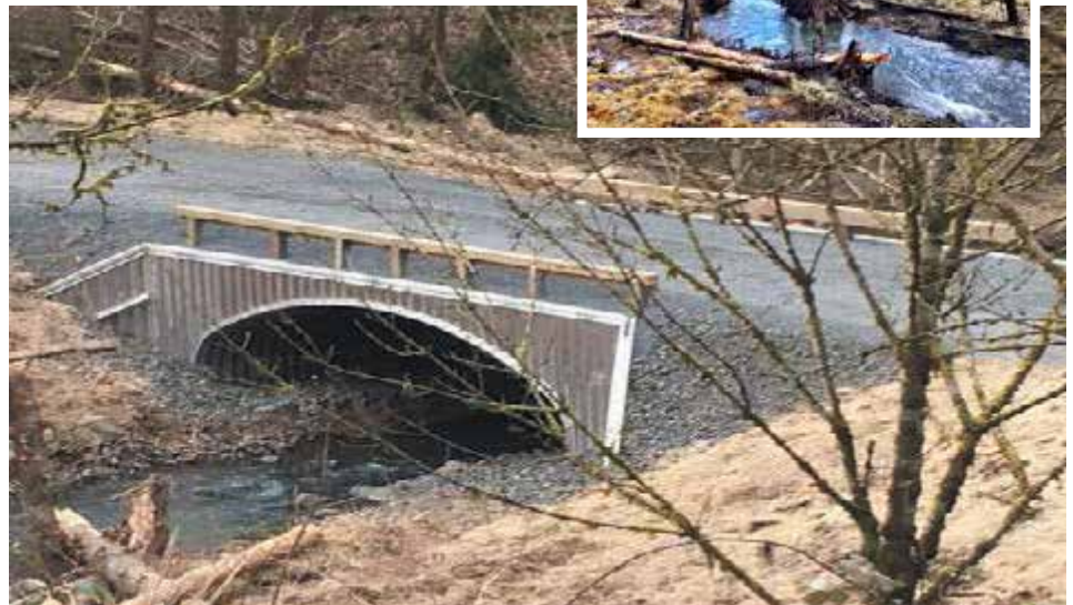
The undersized culvert was replaced with a bottomless arch culvert for better flow, reduced flooding, and improved fish passage. Hills Haven Road was reconstructed.
