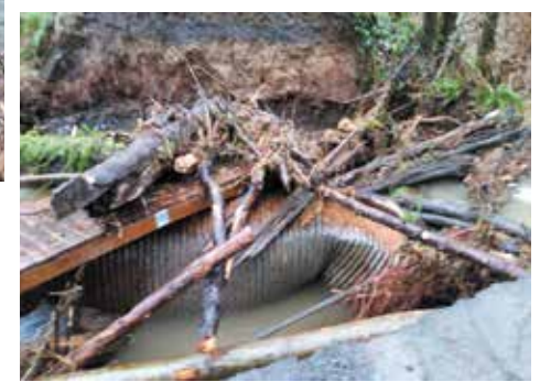
A close up of the culvert after the road had fallen away. Items like small trees and the footbridge from upstream collected on and around the culvert creating a large blockage.
