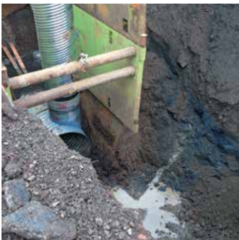
Creating a manhole for access to the new pipe installed on Fox Creek.
