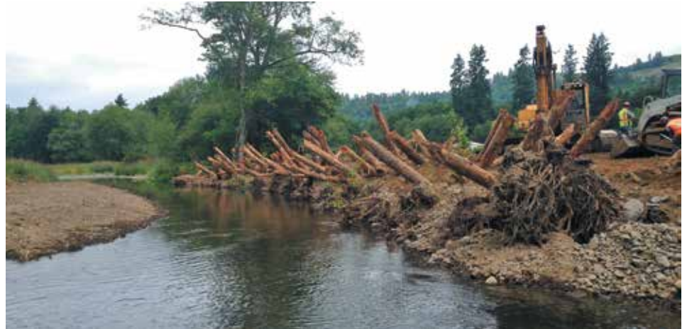
Streambank stabilization project along the Clatskanie River to prevent further erosion and improve flow conditions.
