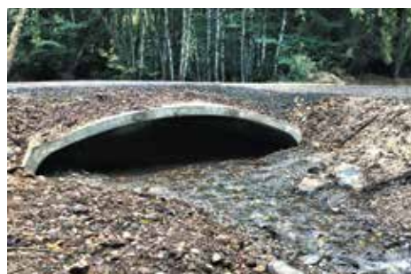
Crossing #5 after construction. Two undersized and ungraded culverts were replaced with 1 large bottomless arch culvert.
