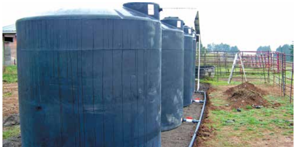
Large rainwater harvest system installed with small grant on a farm in Deer Island.
