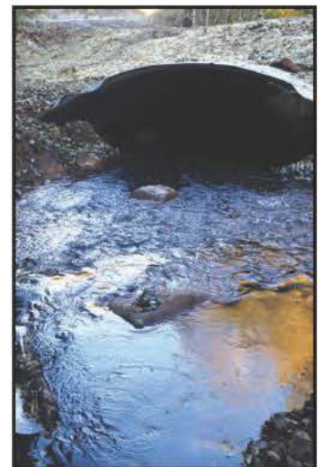
LCRWC partnered with Weyerhaeuser to replace an undersized culvert with a 30' arched, bottomless culvert. Both projects improved fish passage to over 5 miles of habitat.
