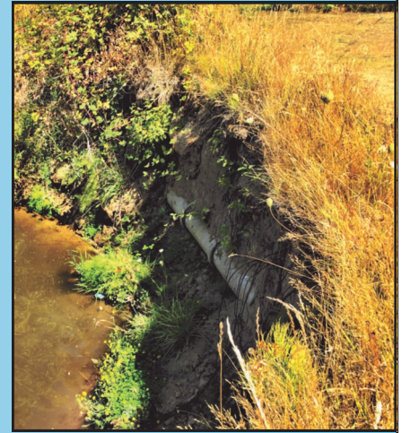
Exposed sewer line during summer low flows.
