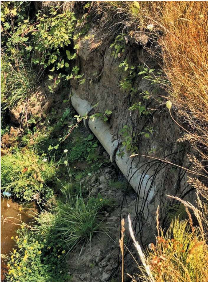
A sewer line running along S. Scappoose Creek was exposed and compromised after severe erosion resulting from the December 2015 storms.
