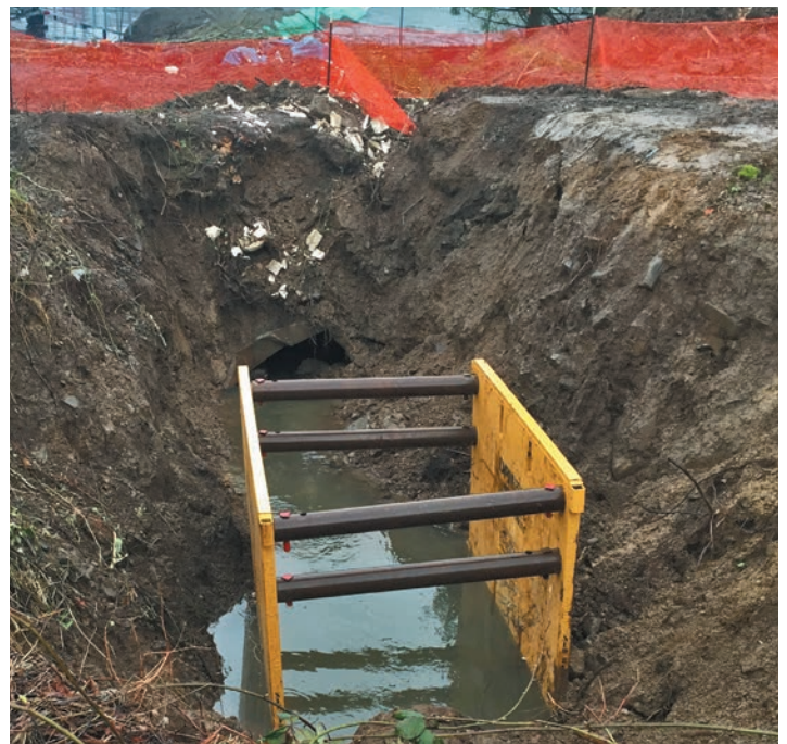
A massive sinkhole formed in the City of Rainier when the underground culvert collapsed during the winter flood.
